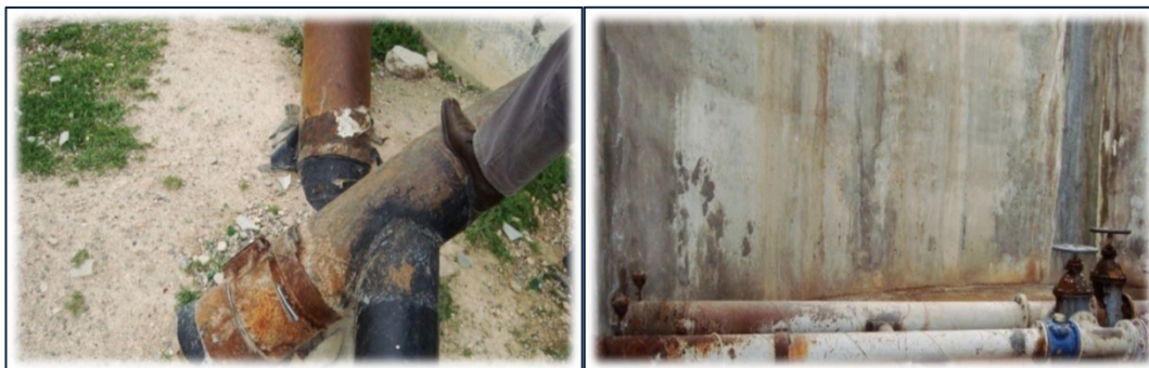
Figure II.23 : Montage et raccordement non professionnel. [82]
